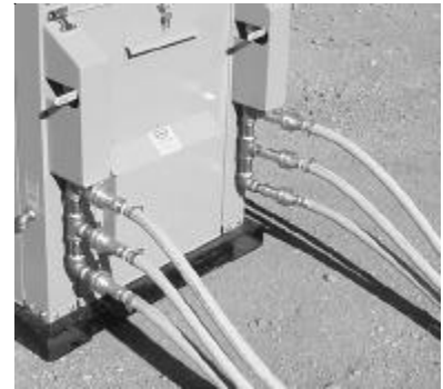
3 - distribution manifold & circulation line heat exchangers
