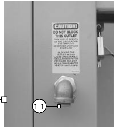
1 - reservoir overflow/vent outlet elbow
