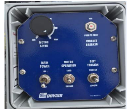
Figure 2 - Hose Reel Control Panel
