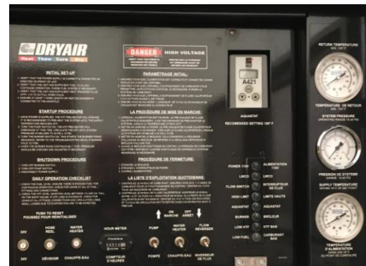
Figure 34 - Control Panel Gauges
