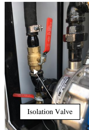
Figure 35 - Pump Isolation Valve
