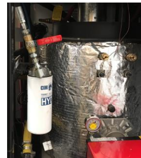
Figure 48 - Fuel Shutoff Valve (Closed)
