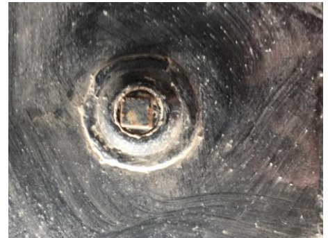
Figure 47 - Secondary Fluid Containment Drain Plug
