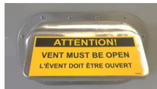
Figure 32 - Air Intake Vent
