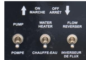
Figure 29 - Control Panel Switches
