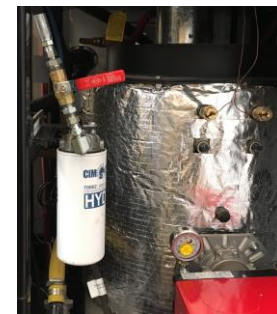
Figure 31 - Fuel Shutoff Valve (Closed)
