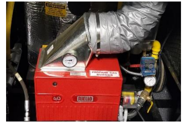
Figure 27 - Propane Gas Burner
