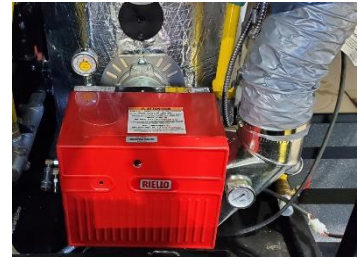
Figure 26 - Diesel/Light Oil Burner
