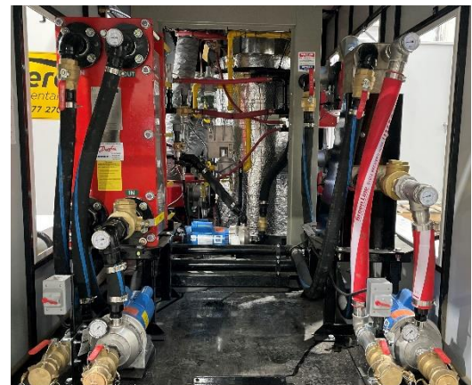
Figure 3 - Plate Heat Exchangers
