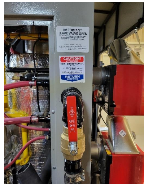
Figure 47 - Glycol Return Valve
