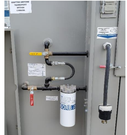
Figure 22 - Fuel Line Valves and Filter
