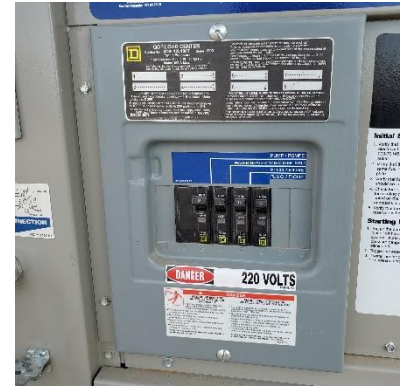
Figure 24 - Pump and Water Heater Switches
