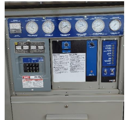
Figure 25 - Control Panel, Temperature Gauges
