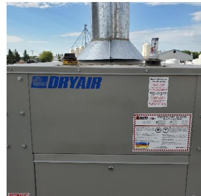
Figure 20 - HTF Level Gauge and Vent
