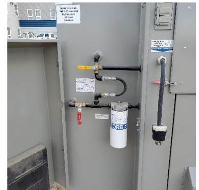
Figure 28 - Fuel Line Valves and Filter
