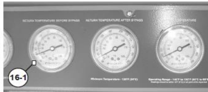
Figure 30-Return Temperature Before Bypass Gauge
