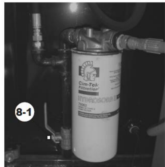
Figure 22-Fuel Supply Valve & Filter
