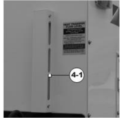
Figure 18-Heat Transfer Fluid Sight Glass
