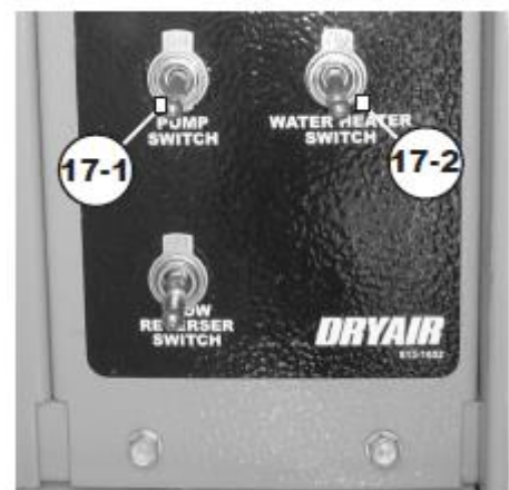
Figure 31-Pump & Water Heater Switch
