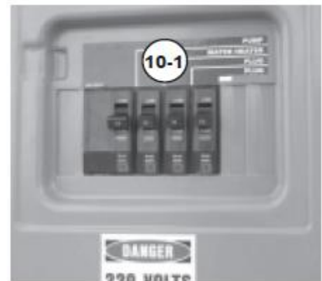
Figure 24-600 GTS Breaker Box
