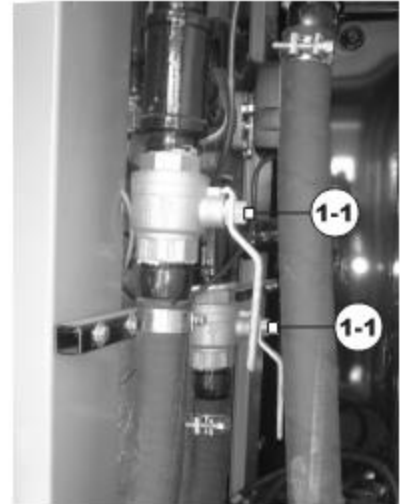
Figure 15-Supply & Return Isolation Valve in the Open Position
