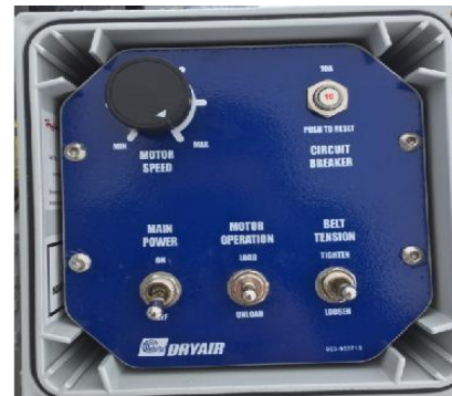
Figure 41 - Hose Reel Control Panel
