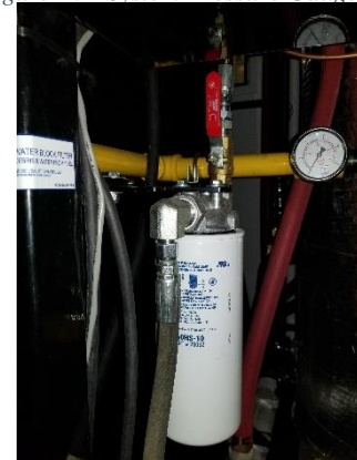
Figure 27 - Burner Fuel Supply Valve and Filter
