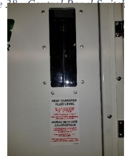
Figure 39 - Glycol Level Gauge
