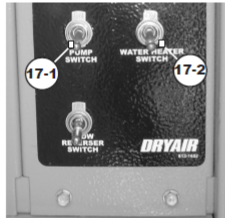
Figure 31-Pump & Water Heater Switch
