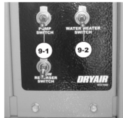
Figure 23-900 GTS Control Panel
