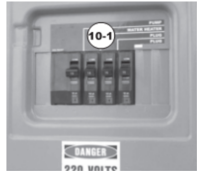
Figure 24-900 GTS Breaker Box
