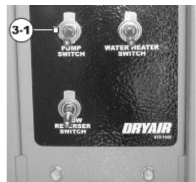
Figure 17-Pump, Water Heater & Flow Reverser Switch
