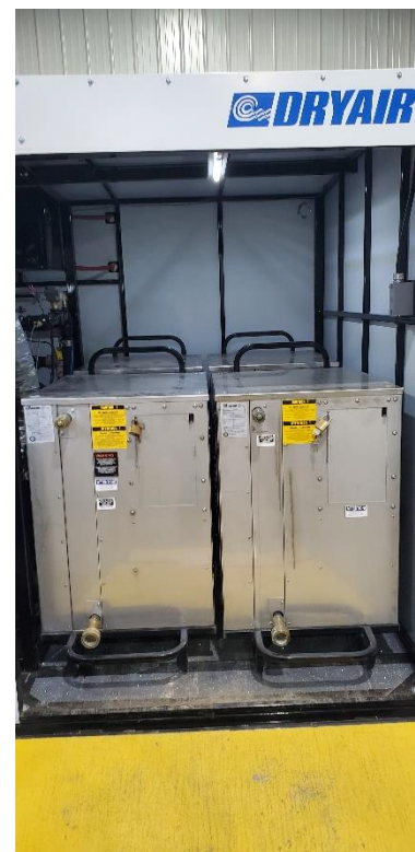
Figure 43 - Storage Bay with 4x ES200 Fan Coils
