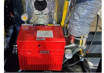
Figure 26 - Diesel/Light Oil Burner
