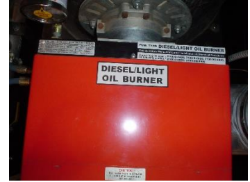
Figure 18 - Diesel/Light Oil Burner
