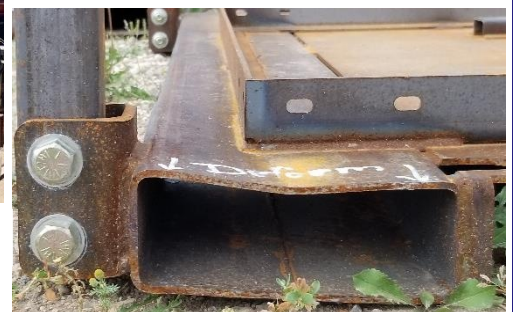
Figure 5. Deformation of the system base near the lifting frame corner post mount bracket.
