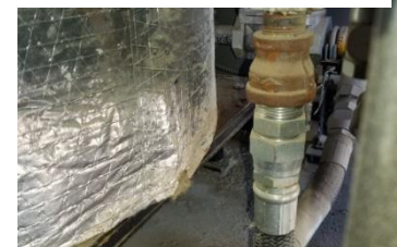
Figure 24 - Gas Supply Hose
