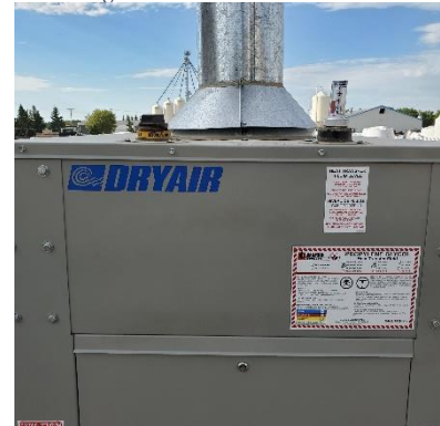
Figure 28 - HTF Level Gauge and Vent
